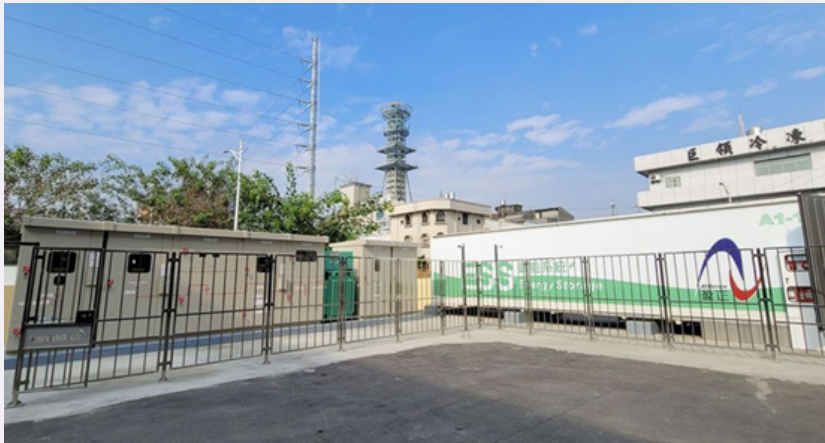
Pintung Plant I ESS 1MW
